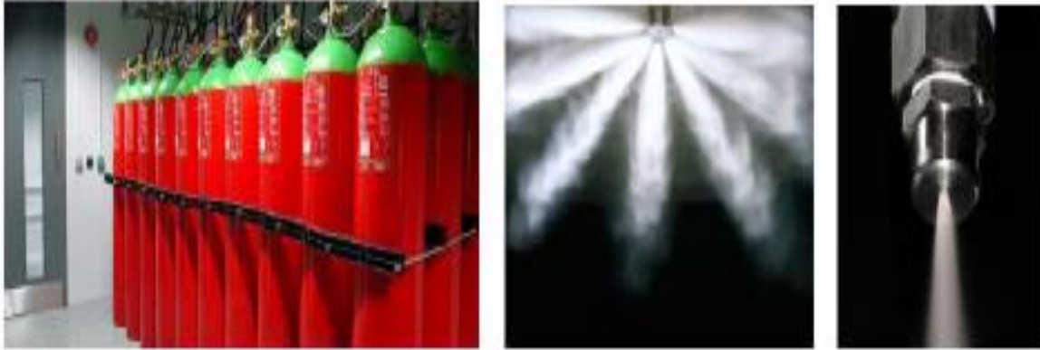
Figure 28: Clean agent systems
